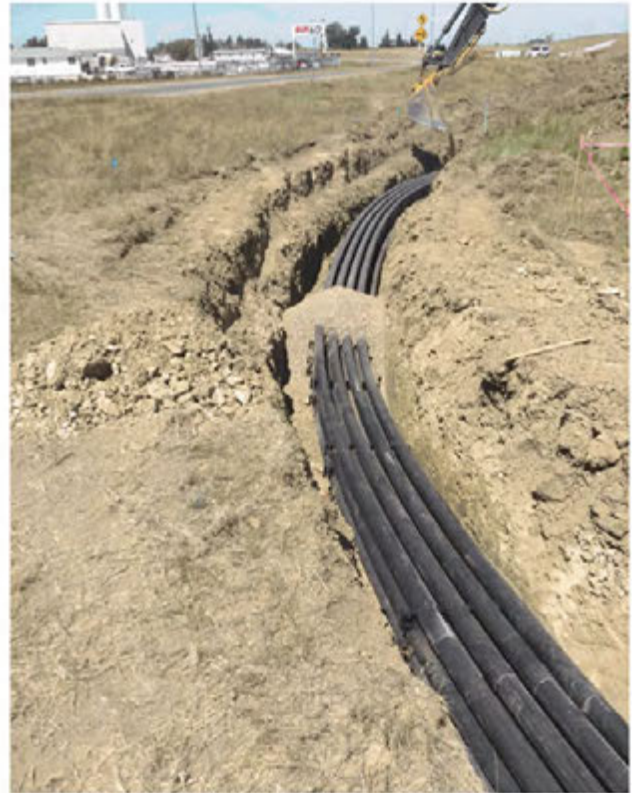
Main Line Feeders
