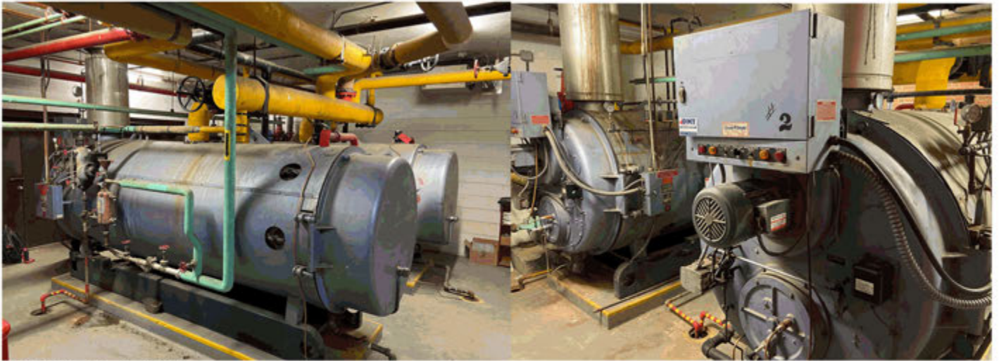
Fritz Sick Centre Boilers
