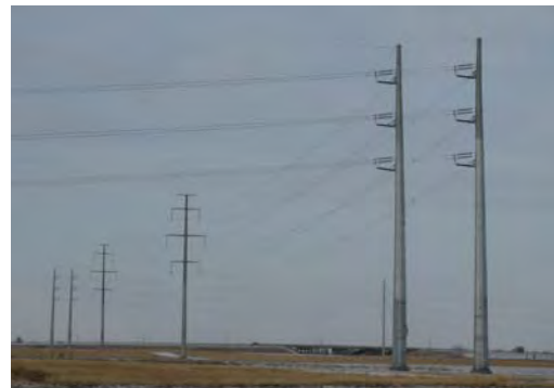
240 kV transmission line in the plan area
